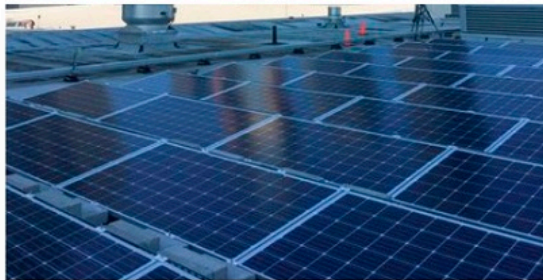
Solar panels, part of 193 solar panels, are seen on the roof of the United Nations headquarters in New York City on September 21, 2019. (LAURA BONILLA CAL/AFP via Getty Images)
